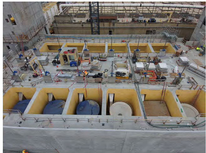
Headworks Grit Separation Units
