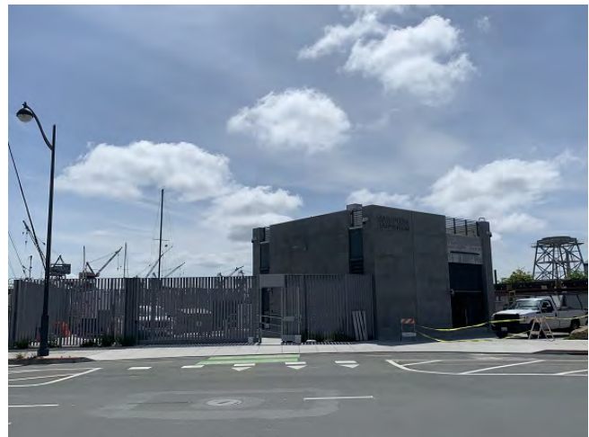
Punchlist items being addressed at Station, including installation of gates and testing of security system.
