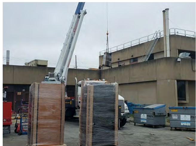
A crane lifting the new DCS server cabinets for installation at Southeast Plant
