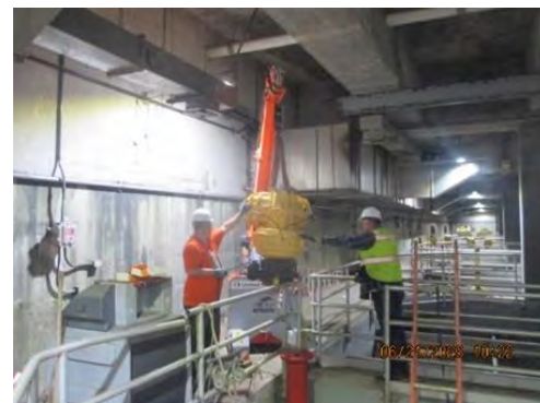
(E) WW-648 OSP Building 042 Primary Clarifier Improvements: Building 042 Clarifier No.1 Contractor continues install of effluent butterfly valve and pneumatic actuator installation.
