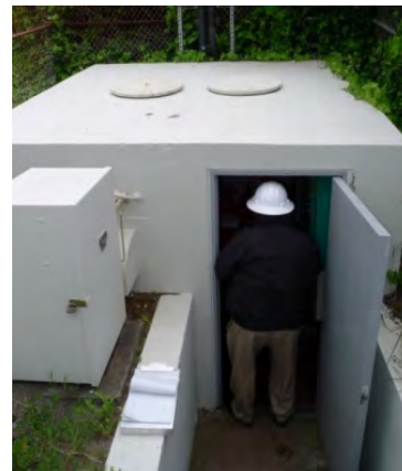
Seacliff Pump Station No. 1
