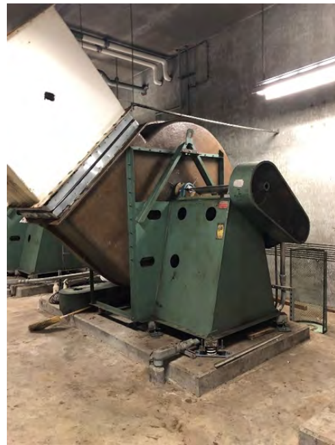
At building 011 exhaust fan room, as-found condition of existing exhaust fan assembly identified for replacement.
