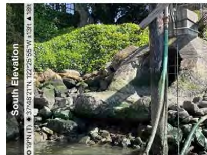
Damaged rip-rap under and around Laguna CSD.
