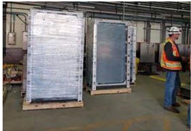
DCS server cabinets delivered at Northshore Pump Station
