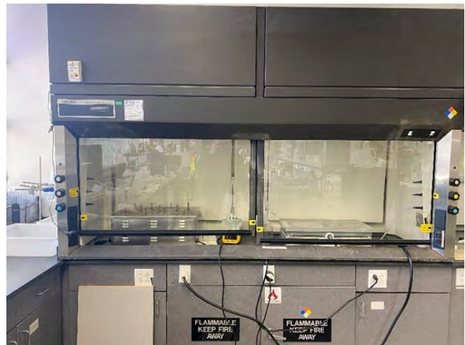
Building 930 laboratory, as-found condition of existing laboratory fume-hood assembly identified for replacement.
