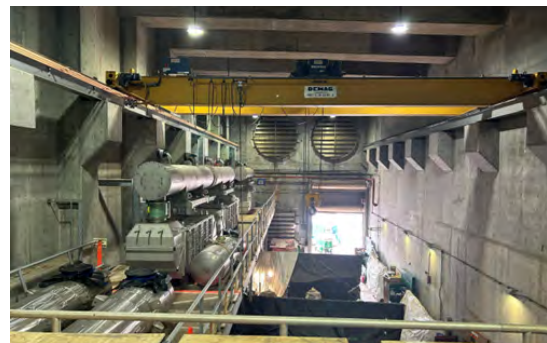
At building 800 cogeneration engine room, the Contractor continues installation of electrical and mechanical equipment.
