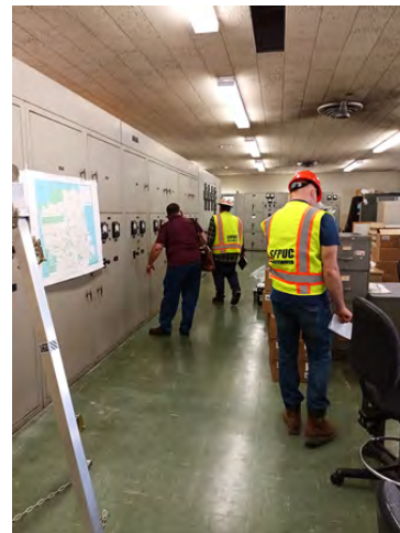
WWE staff and design team surveying existing obsolete electrical equipment at NPF 930 Administration Building.
