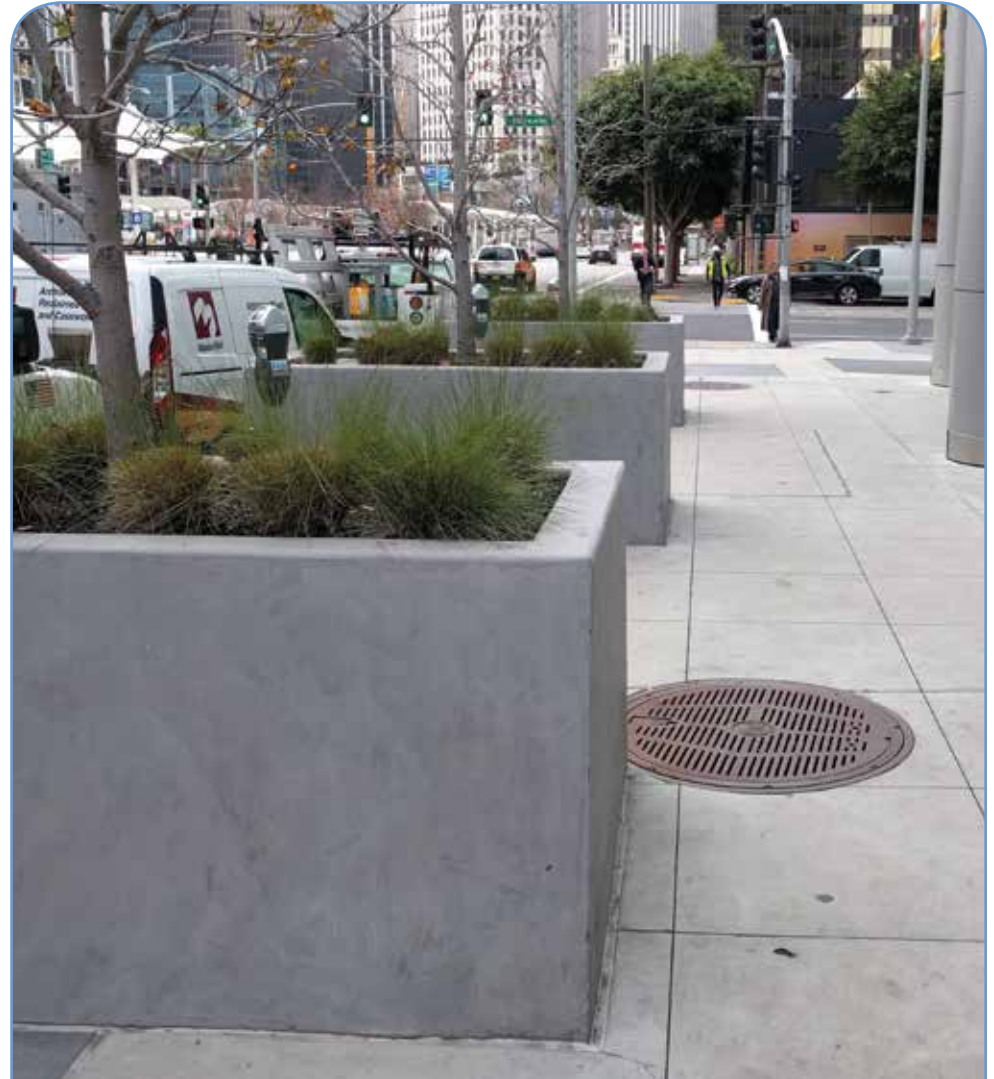
Raised planter boxes (such as the ones pictured) are considered permanent structures, but may be allowable with adequate spacing (Standard W9.a.i and Detail APS WS9.1).
