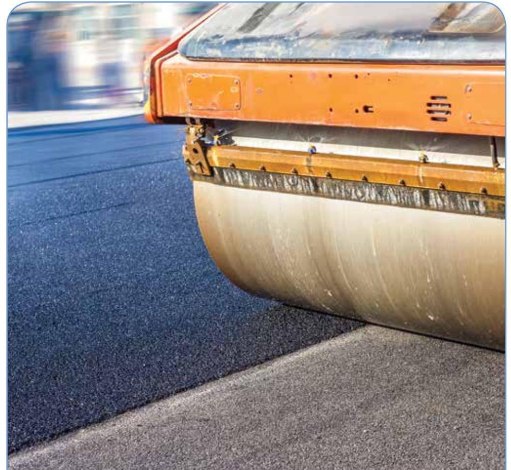
Paving above and around SFPUC assets protects those assets from traffic loads.
