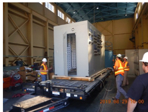
New Motor Control Board at Holm Powerhouse
