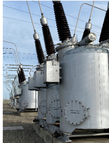
Old Oil Circuit Breakers to be Replaced
