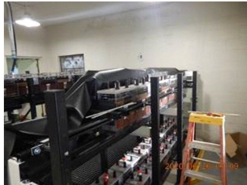
Warnerville New Direct Current Battery Bank
