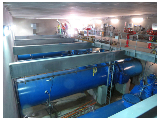
SJPL#1-4 with isolation valves within Tesla Valvehouse
