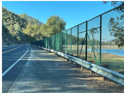
Installation of Chain link fences and gates along Highway 49 are in progress
