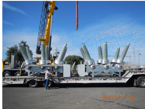
Oil Circuit Breakers
