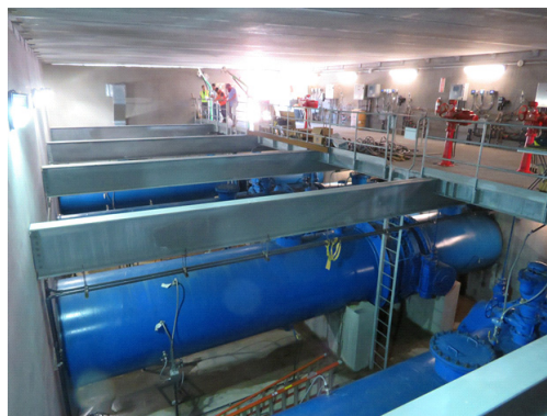
SJPL#1-4 with isolation valves within Tesla Valvehouse
