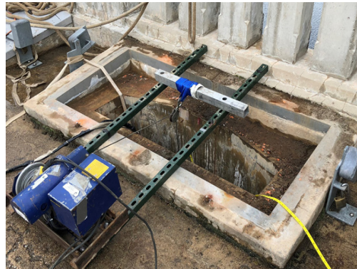
Bulkhead gate slot at top of dam and setup for underwater camera inspection
