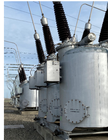
Oil Circuit Breakers
