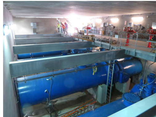
SJPL#1-4 with isolation valves within Tesla Valvehouse
