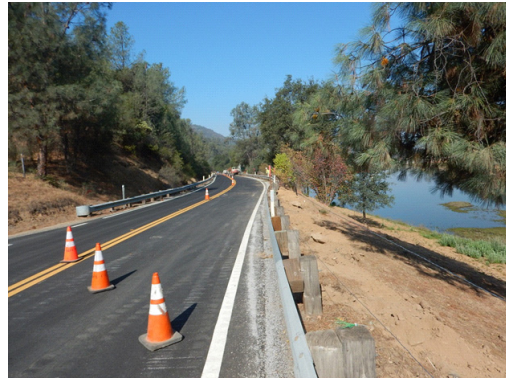
Construction has started along Hwy 49 for the Moccasin Security Perimeter Fence Project; road traffic control is in place.
