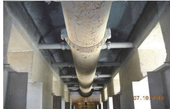
Pipe Corrosion in Air Scour Tank
