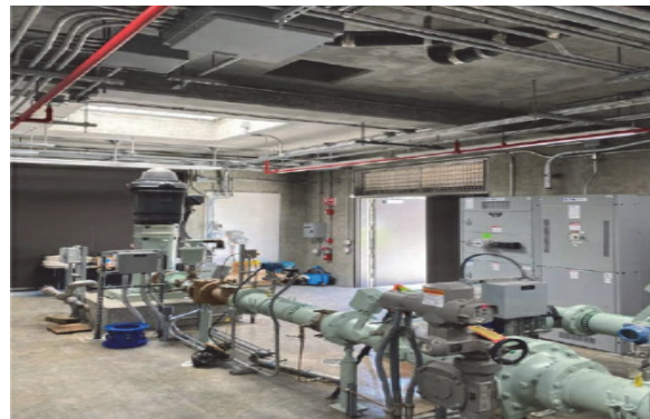
Typical well site
