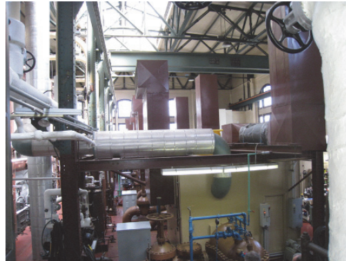
Interior view of PS2 showing a pump, valves, engine sound enclosure and exhaust, and building structural members
