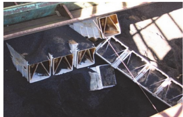
Filter underdrain failure
