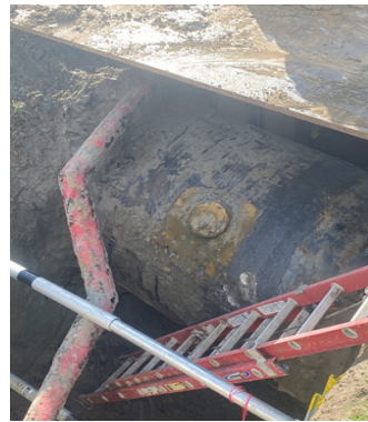
Additional pothole location showing previous repair
