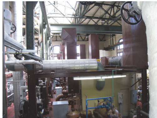
Interior view of PS2 showing a pump, valves, engine sound enclosure and exhaust, and building structural members
