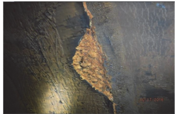
Typical Lining Defect
