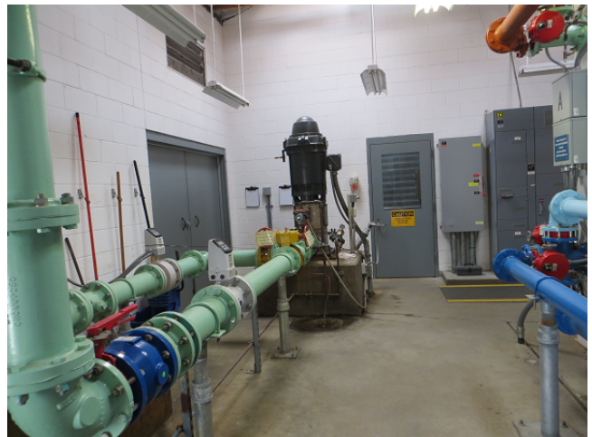
Typical Well Station Equipment
