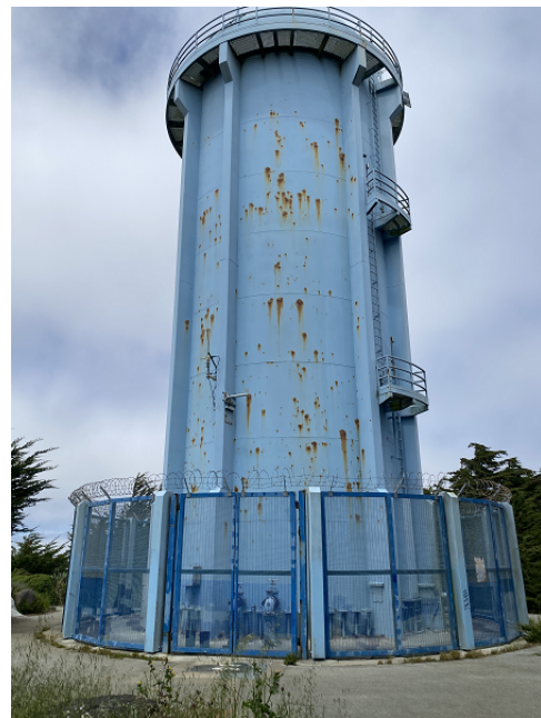
Premature Coating Failure and Corrosion at La Grande Tank
