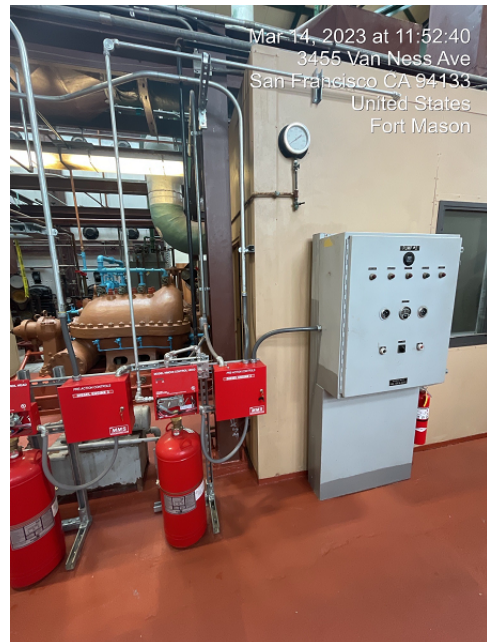
EFWS Pump Station No. 2
