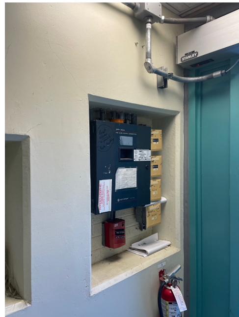
Existing Fire Alarm Control Panel to be Upgraded
