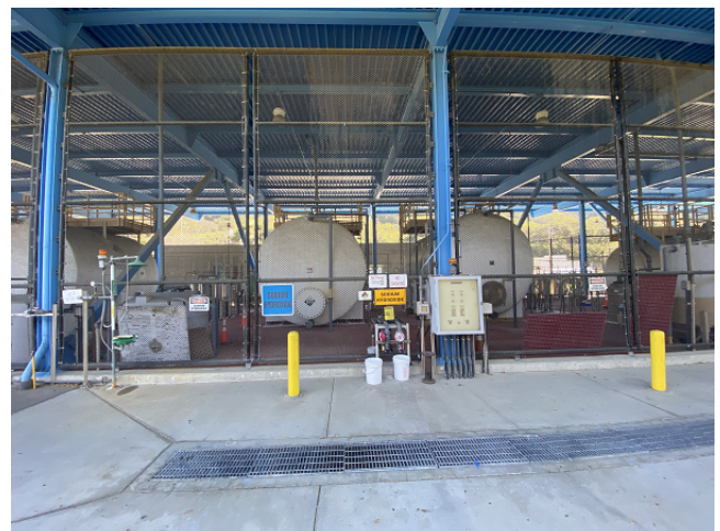
Sunol Valley Chloramination Facility Sodium Hydroxide Tanks
