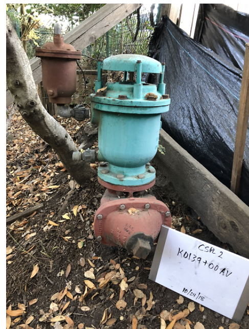
Typical Air Valve to be Upgraded
