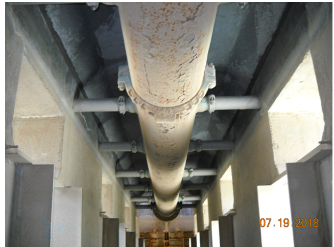
Corrosion on Existing Air Scour Pipeline
