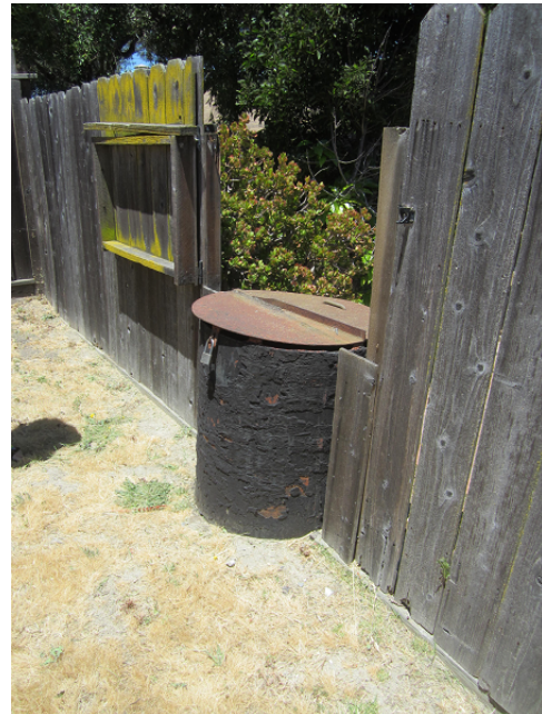
Typical Air Valve to be Upgraded
