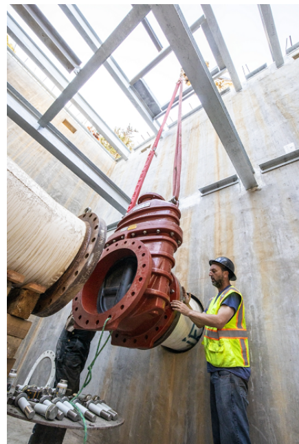
Installation of 24-inch Gate Valve inside the Valve Control Vault at College Hill Reservoir
