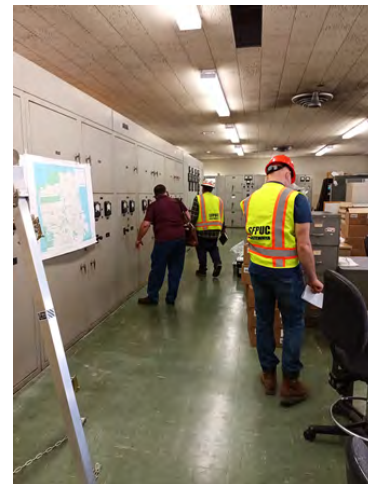
WWE Staff and Design Team Surveying Existing Obsolete Electrical Equipment at NPF 930 Administration Building
