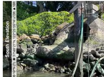
Damaged Rip-Rap Under and Around Laguna CSD
