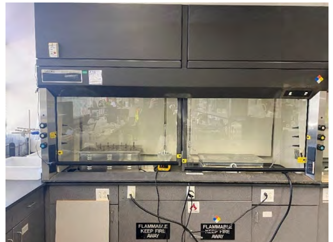
Existing Laboratory Fume-Hood Assembly Identified for Replacement at Building 930 Laboratory.
