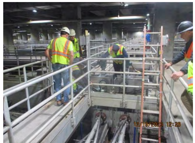
Project (E) WW-648 OSP Building 042 Primary Clarifier Improvements, Tank No. 5 helical scum skimmer installation in December 2023.
