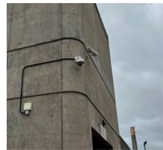
Existing Cameras on a Building at SEP
