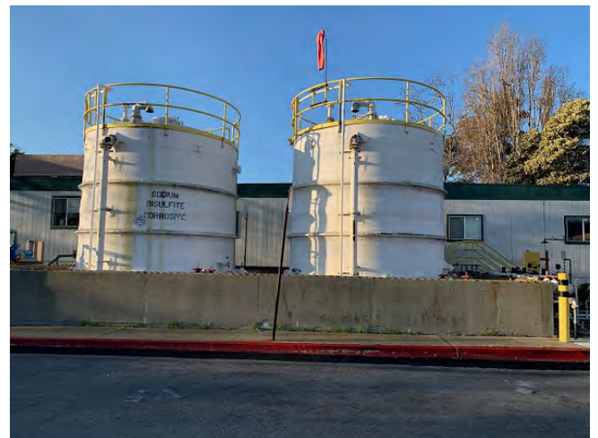
Existing Sodium Bisulfite Tanks
