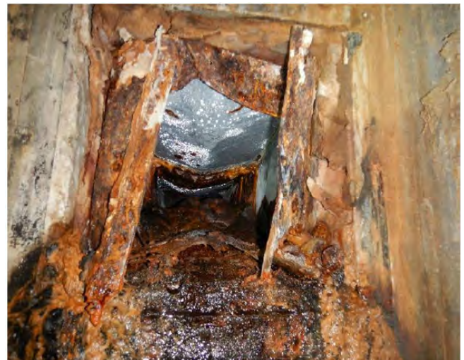
HVAC Ducting Corrosion due to Water Intrusion
