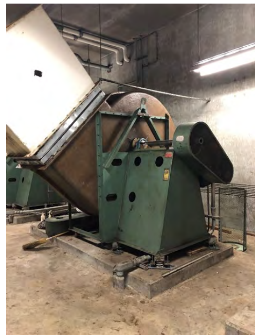
Existing Exhaust Fan Assembly Identified for Replacement at Building 011 Exhaust Fan Room.
