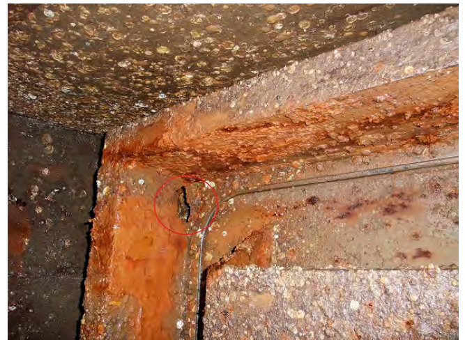
Brannan CSD Existing Damaged Butterfly Discharge Valve
