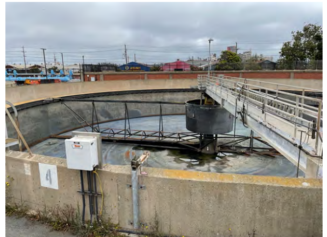
One of the Secondary Clarifiers To be Replaced Under This Project
