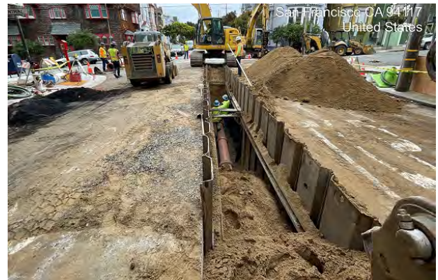
Open trench excavation and replacement of 12-inch main sewer on Page Street, San Francisco
