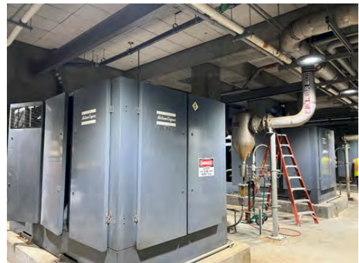
As-found Condition of Existing Pressure Swing Absorption (PSA) Oxygen Generation Process Equipment
