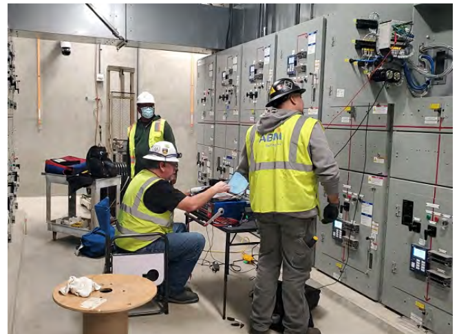
Relay Testing of Primary Switchgear
