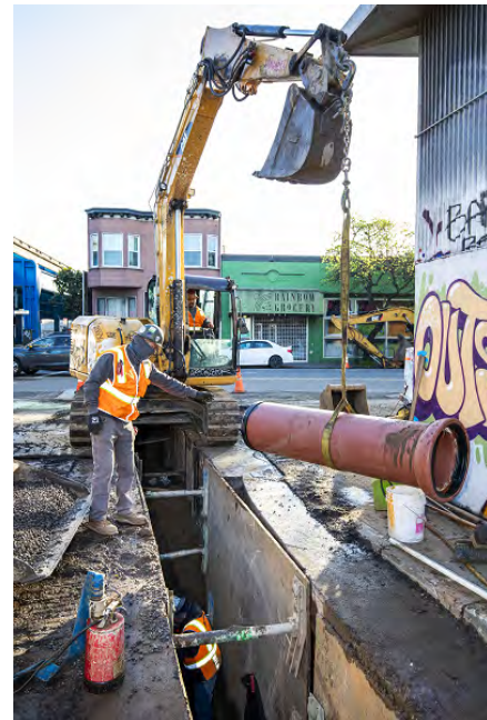
Installation of new combined sewer pipe on Erie Street as part of the WW-719A contract
