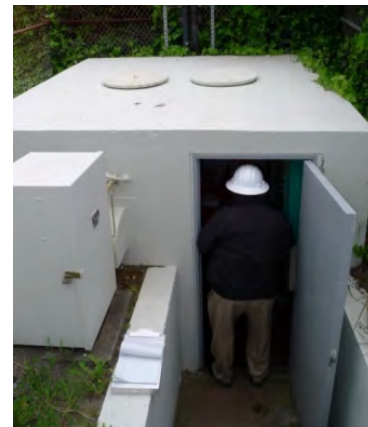
Seacliff Pump Station No.1
