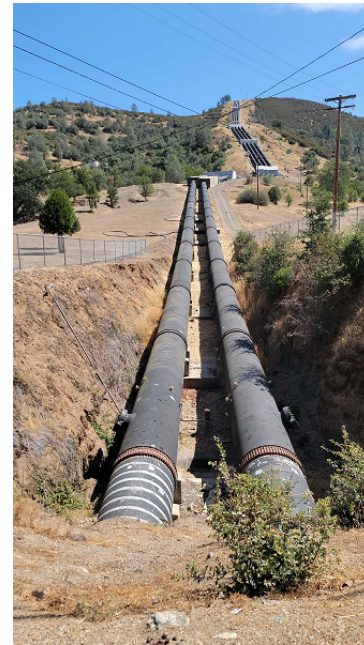
Moccasin Bypass Penstock Tie-in Point
