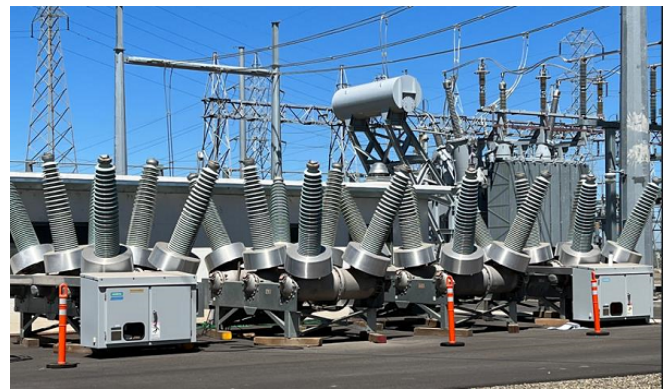
Four 230 kV SF6 Circuit Breakers to be installed during Phase 2
