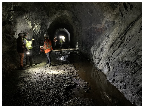
Site visit to evaluate the existing plug at Hetch Hetchy Adit within the Canyon Tunnel
