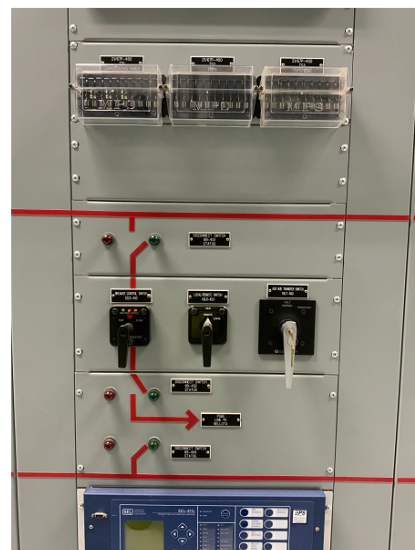
TOP: Warnerville Substation South Yard BOTTOM: Warnerville Substation Protection and Control Relay Panel
