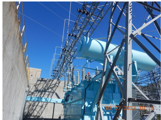
GSU Final Connections on High and Low side [HH-1003R]
