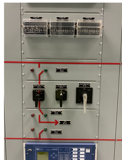
TOP: Warnerville Substation South Yard
