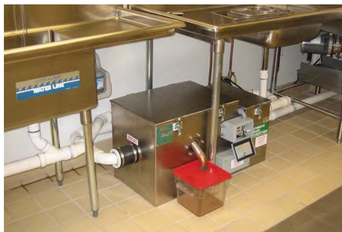
Figure 4. Example of an installed automatic grease removal device. Source: The Wastewater Solutions Update
