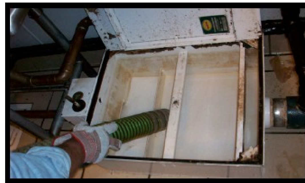
Figure 5. Example of a trap being cleaned by a contractor. Source: Bay Area Pollution Prevention Group
