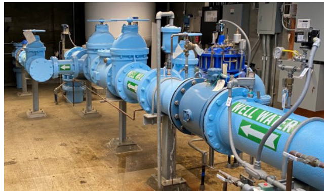
Golden Gate Park groundwater facility (Source: C. Ripley, 2020)
