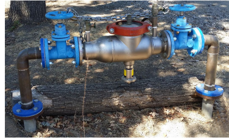
Example of a Backflow Prevention Assembly
