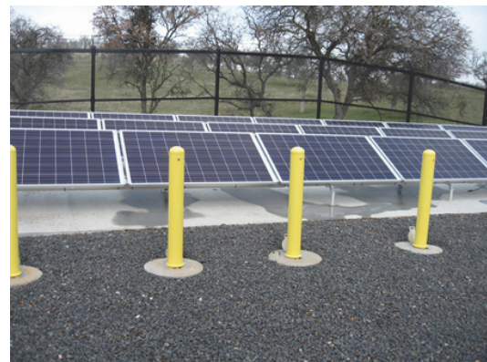
Oakdale Valve House No. 4 Solar Facilities
