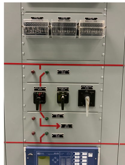
TOP: Warnerville Substation South Yard BOTTOM: Warnerville Substation Protection and Control Relay Panel
