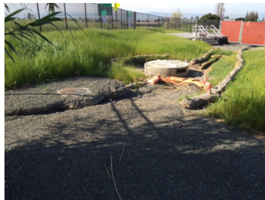
Erosion Across ROW Due to Caltrans Drainage Pipe
