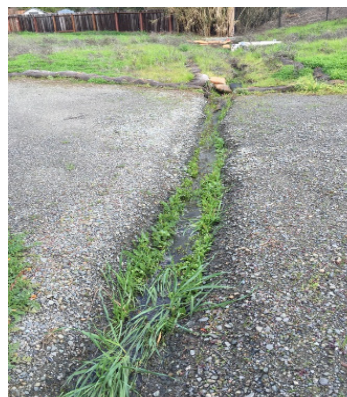
Erosion Across ROW from Caltrans Drainage Linet
