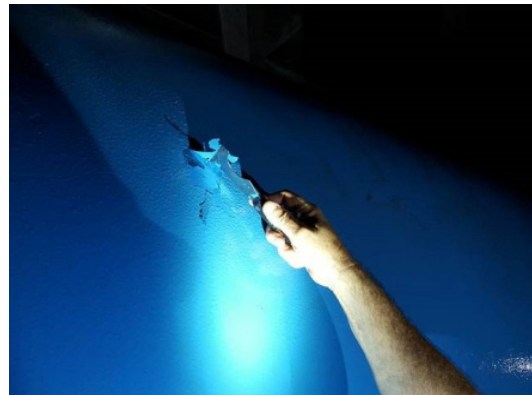
BDPL#3 Coating Peeling Away from Pipe
