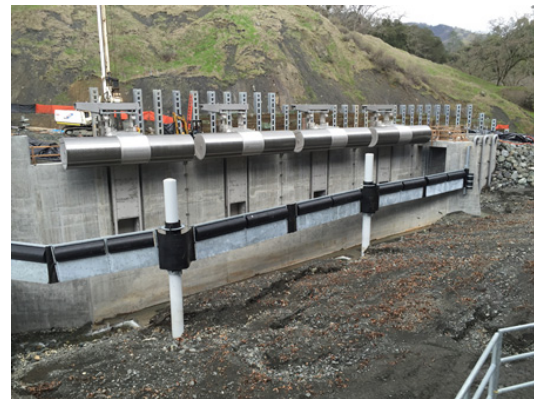
Fish Screens Installed at the Intake Structure
