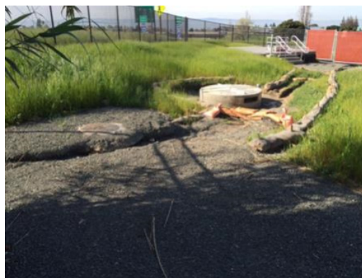
Erosion Across ROW Due to Caltrans Drainage Pipe
