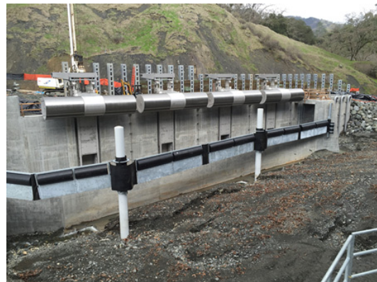
Fish Screens Installed at the Intake Structure
