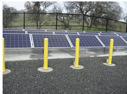
Oakdale Valve House No. 4 Solar Facilities
