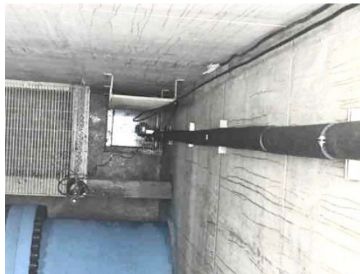
Ventilation Fan and Control Panel at the Articulated Vault
