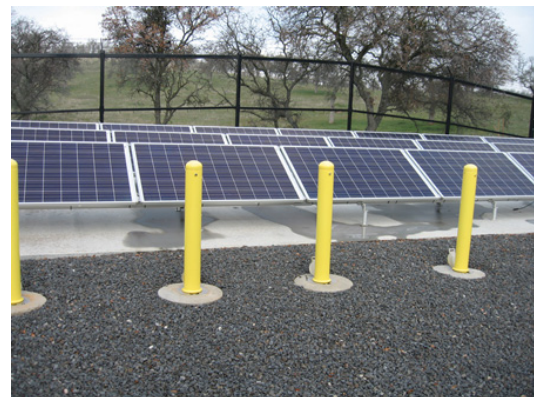
Oakdale Valve House No. 4 Solar Facilities
