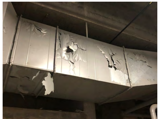
OSP Building 200 Existing Deficient Ductwork
