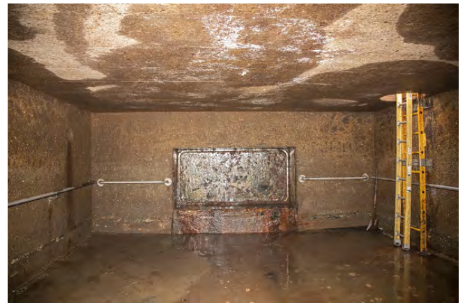
Brannan CSD Existing Damaged Butterfly Discharge Valve
