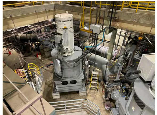
Dry Weather Pump No. 1 Installed and Painted
