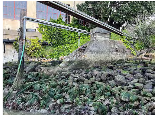
Damaged Rip-Rap Under and Around Laguna CSD
