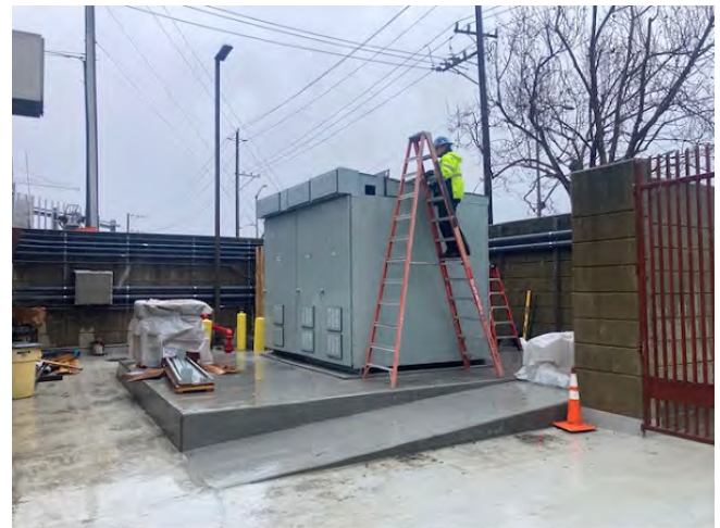
Switchgear at Bruce Flynn Pump Station
