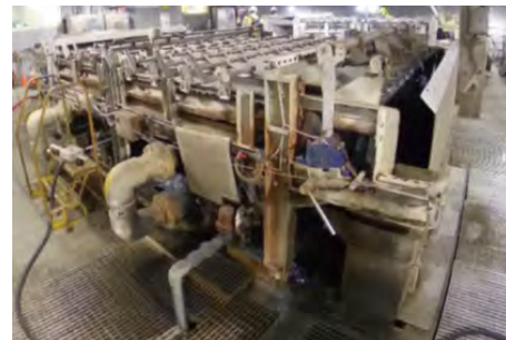
OSP Building 011 Existing Deficient Gravity Belt Thickener Wastewater Process Equipment
