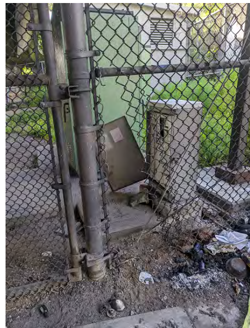
Security Issues at Cesar Chavez Pump Station
