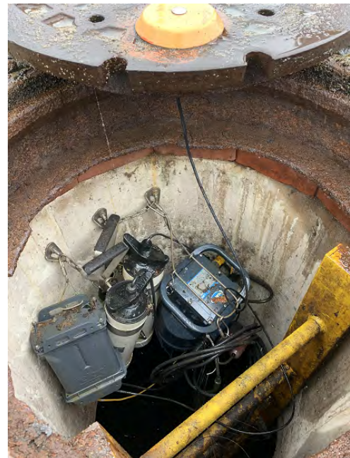
Existing Field Instrumentation Equipment Installed in a Sewer Manhole
