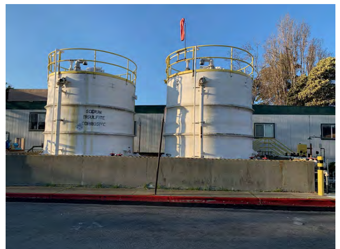
Existing Sodium Bisulfite Tanks
