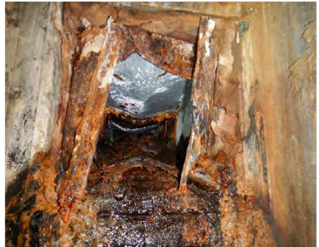
HVAC Ducting Corrosion Ddue to Water Intrusion
