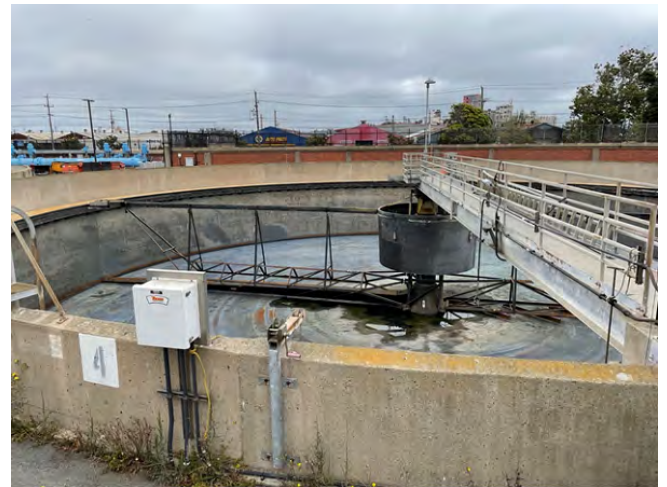
One of the Secondary Clarifiers To be Replaced
