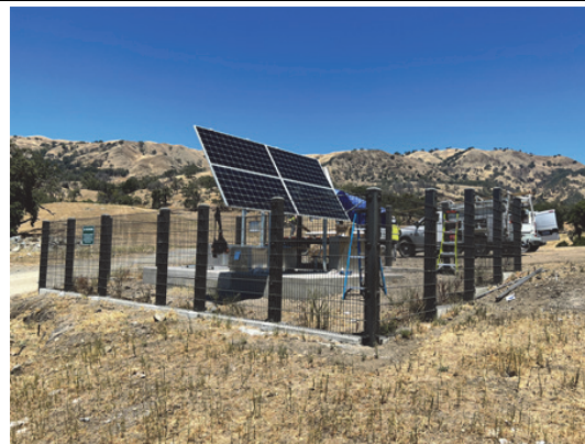
Photovoltaic System, Backup Generator and Propane Tank
