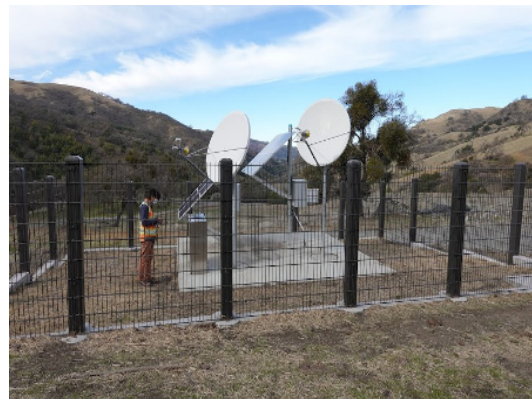
VSAT System Upgrade Site
