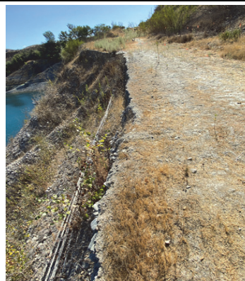
Erosion Along Existing Access Road
