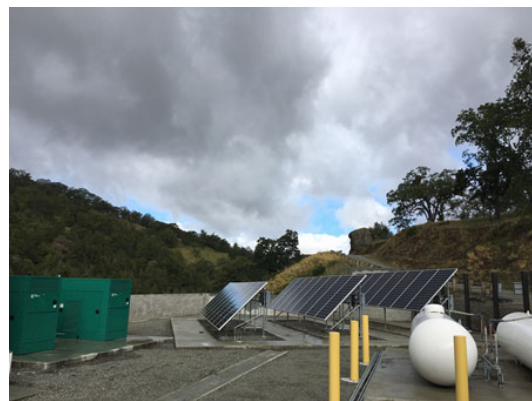
PV System, Backup Generator and Propane Tank
