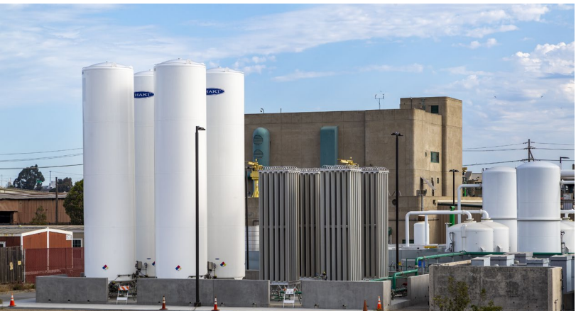
SEP Cryogenic Oxygen Plant Completion
