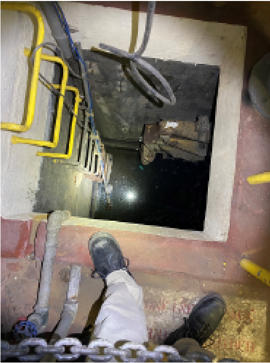
Wet Well of Pump Station
