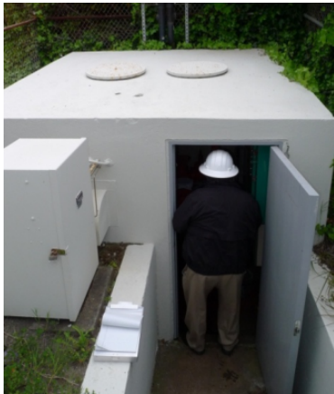
Seacliff Pump Station No.1
