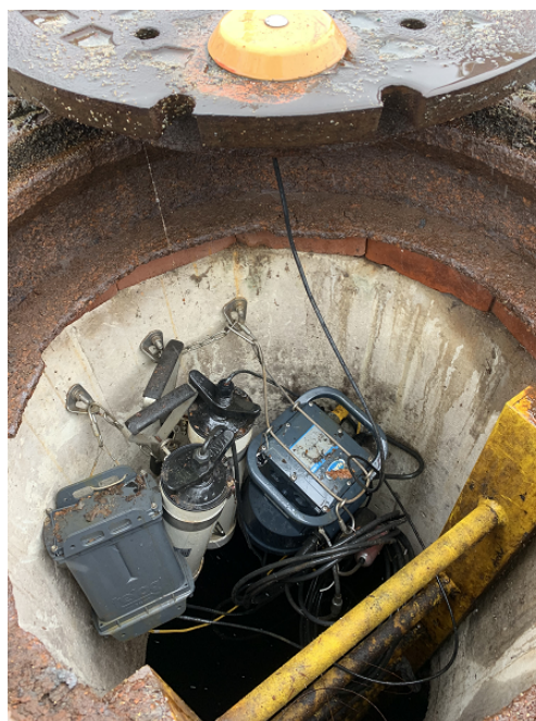
Existing field instrumentation equipment installed in a sewer manhole
