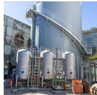
The Gas Holder Tank Building 741 digester gas piping and siloxane removal system.
