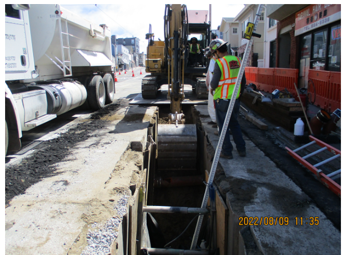
Segment B: Contractor carefully excavating soil to prepare for sewer pipe installation
