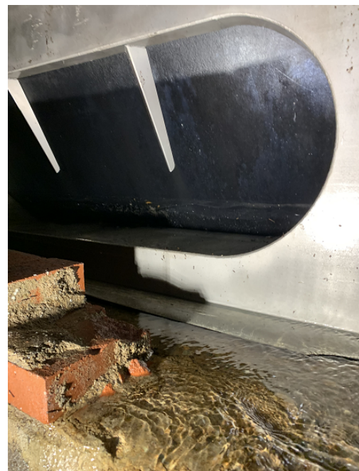
Leaky backflow preventor valve at Baker CSD.
