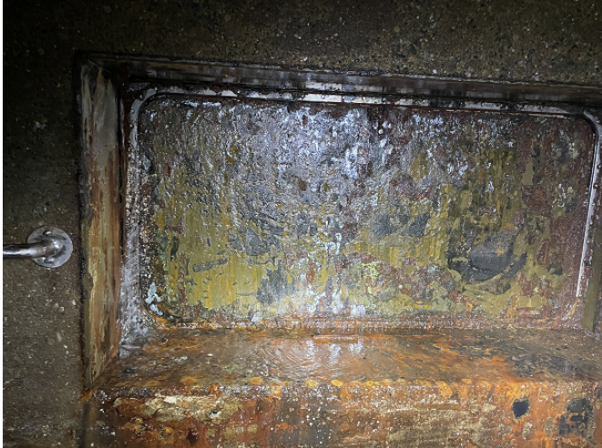
Brannan CSD butterfly valve stuck in place.
