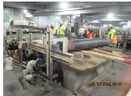
Selective equipment demolition to GBT No. 1; this work is expected to be completed prior to the project contract work commencing on the replacement of GBT No. 2 and GBT No. 3.
