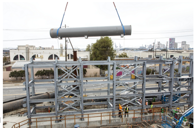
Drill Pier work for Pipe Rack in vicinity of Union Pacific Railroad Right-of-Way
