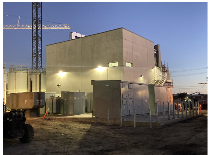
Primary Switchgear Bldg. at Night
