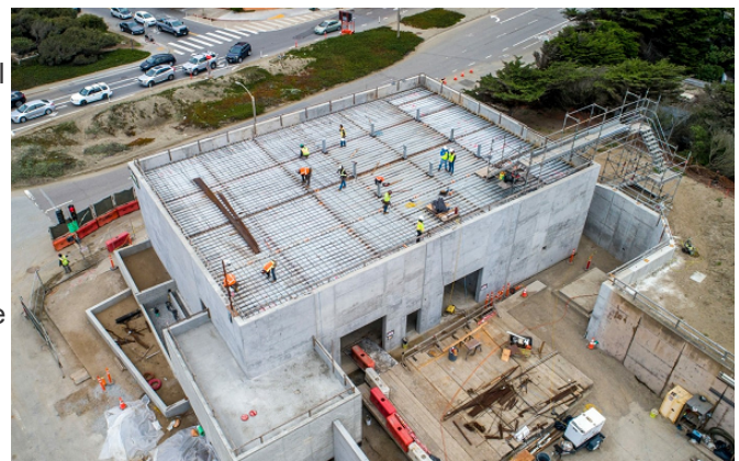
Contractor installing rebar reinforcement at new Electrical Building Roof as of September 2022.
