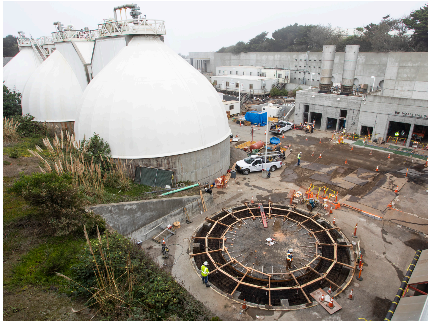
Digester Gas Utilization Upgrade Project - Concrete pour on future location of gas holder tank that will hold excess digester gas.
