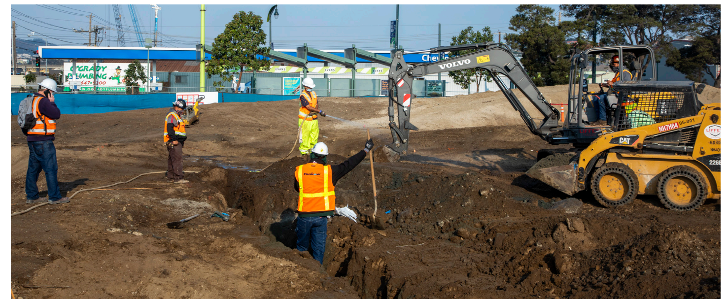
Digging a trench to install conduit at the new Southeast Community Center at 1550 Evans Avenue
