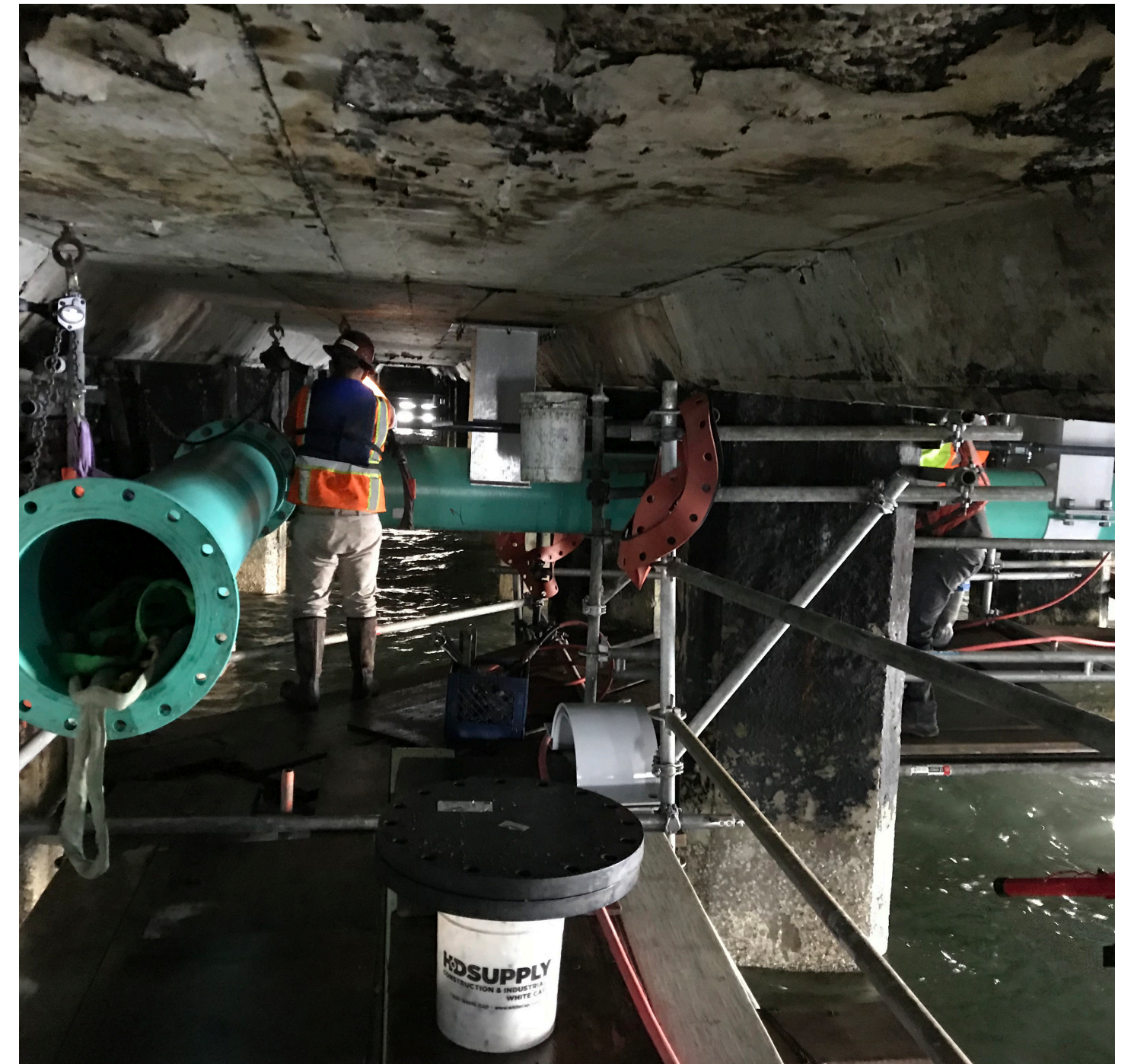
North Point Facility Outfall Rehabilitation Project: installation of outfall structure beneath pier 35
