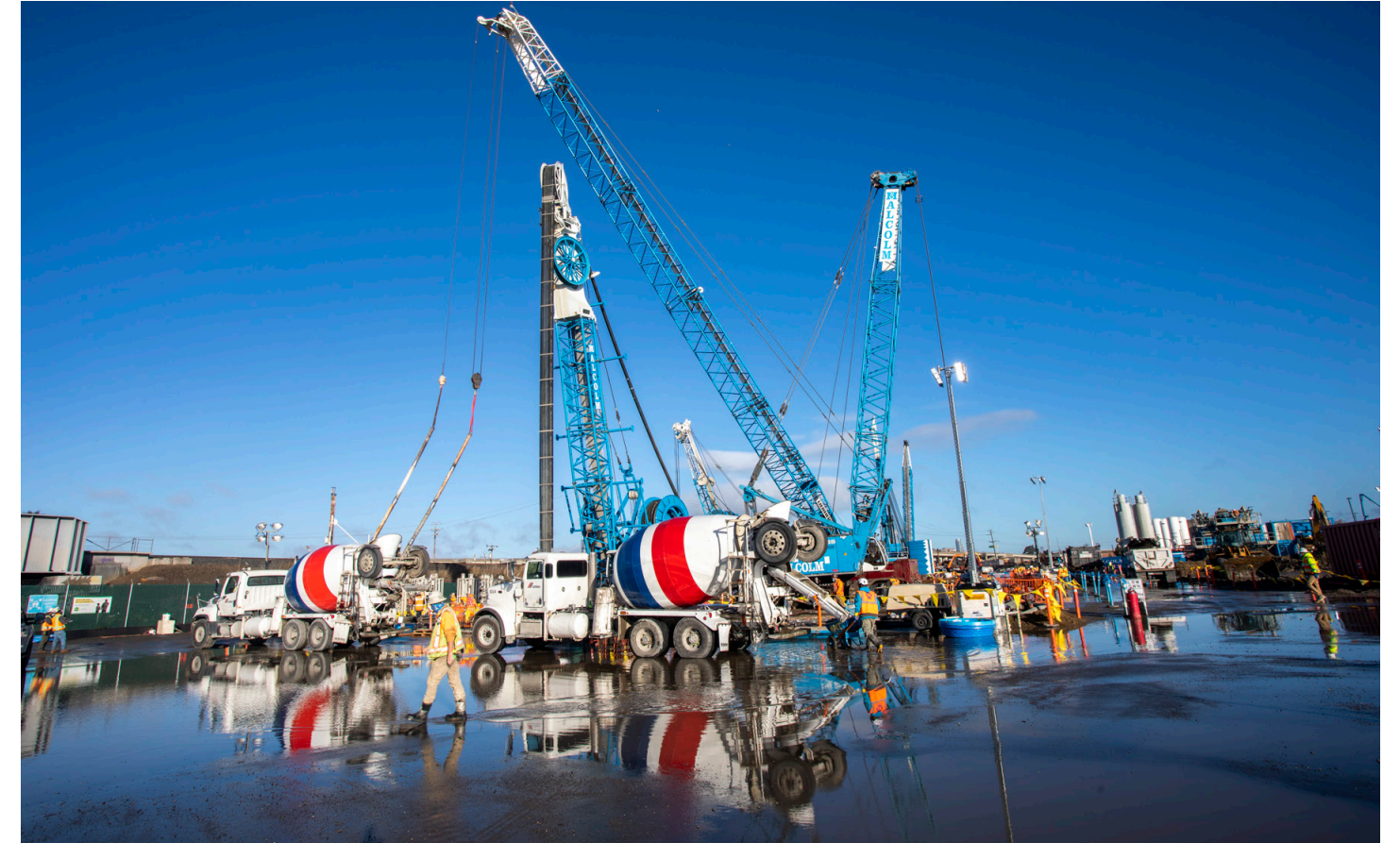
Biosolids Digester Facilities Project: Hydro Cutter, machinery used to build the slurry wall. The slurry wall will be 150-ft deep and cuts off the groundwater. Kurt Cutshaw, Malcolm Hydro Cutter Operator
