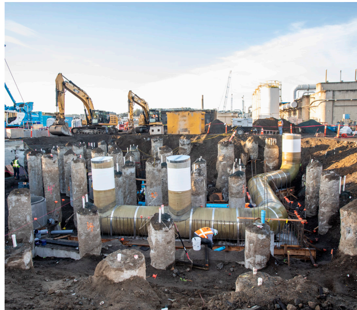
Southeast Wastewater Treatment Plant, Headworks Facility Project: Installation of subsurface pipework around foundation piers
